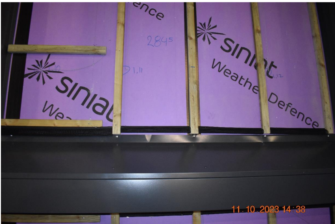
Photo No. 16 The Nordland snow catch pipes were put between the wall and the claddings on the top and bottom of the horizontal flame deflector.
