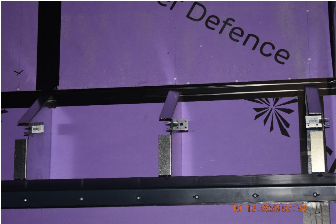
Photo No. 9 Bracket profiles were cut at the front upper side.
