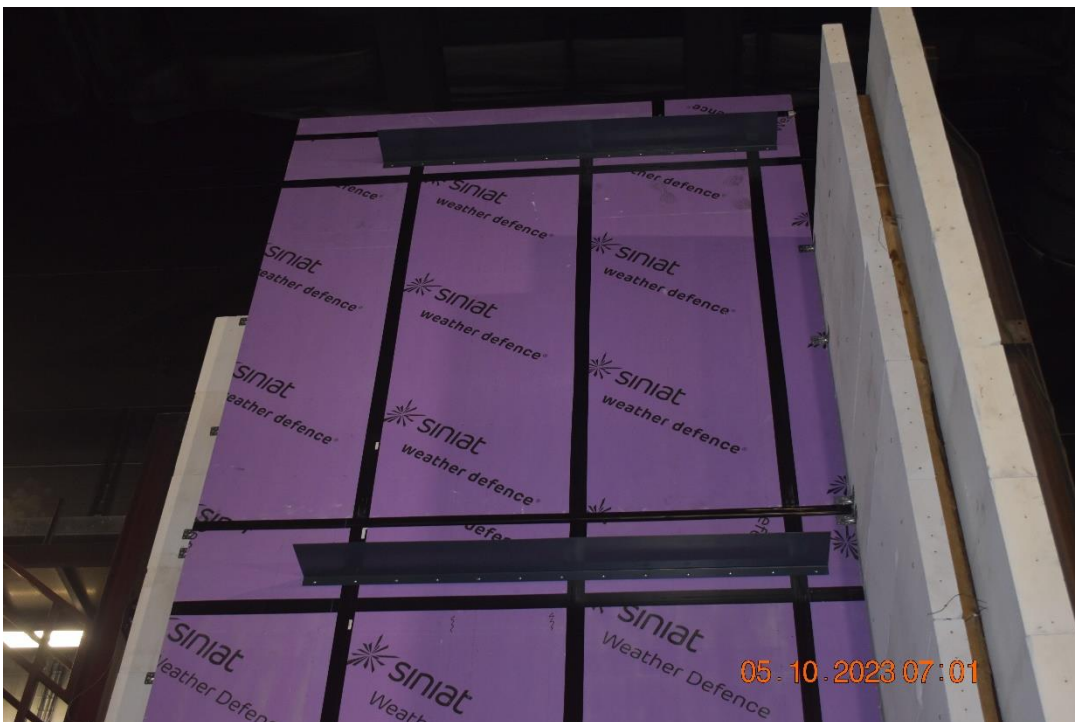
Photo No. 6 Flame deflectors mounted horizontally.
